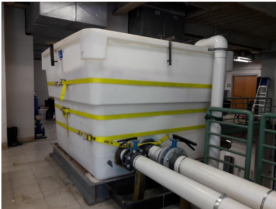
Figure 2.6 The head tank system with pipes (Image by author)
